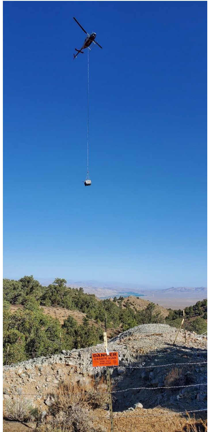
Picture 4 – Helicopter sling line aided delivery of closure supplies at WRSP permanent closure project, Lyon County, Nev.
